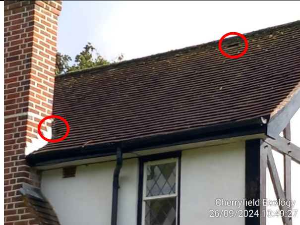
Figure 9: Example of gaps in the roofing tiles
