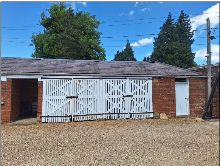
Slatted Doors to Machine Store Image
