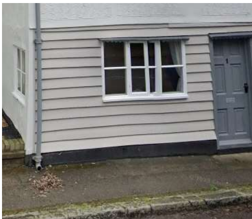
Existing feather edged boarding.
