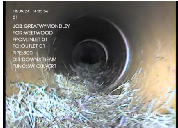
Photo: 1_9A 7.4m, Settled deposits, other, 20% cross-sectional area loss, Start Remarks: Grass / straw
