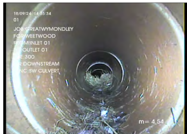
Photo: 1_5A 4.7m, Joint displaced, medium
