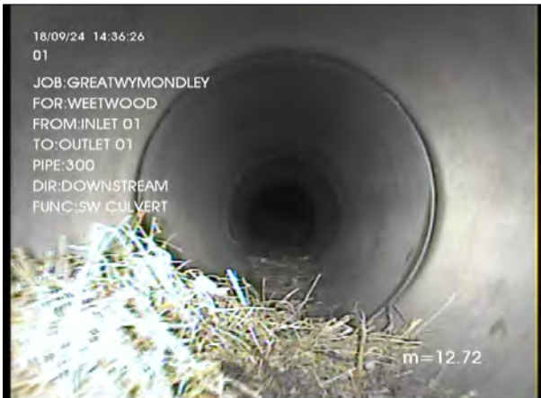
Photo: 1_12A 12.5m, Settled deposits, other, 25% cross-sectional area loss Remarks: Grass / straw
