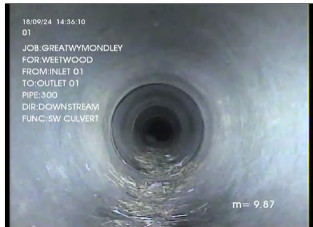
Photo: 1_11A 10m, Settled deposits, other, 5% cross-sectional area loss, Start Remarks: Grass / straw
