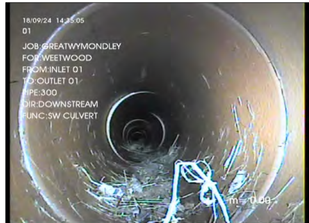
Photo: 1_3A 0m, Settled deposits, fine, 15% cross-sectional area loss, Start Remarks: Silt and grass / straw
