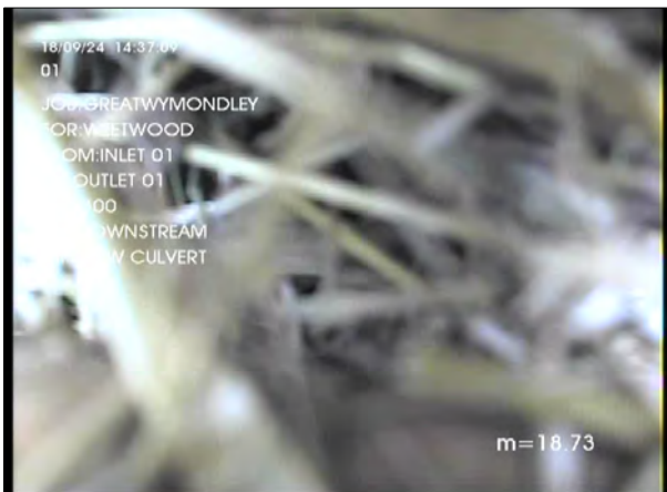
Photo: 1_16A 18.73m, Survey abandoned Remarks: Unable to pass grass / straw build up.
