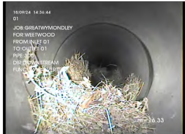
Photo: 1_14A 16.3m, Settled deposits, other, 50% cross-sectional area loss, Start Remarks: Grass / straw
