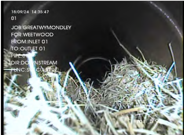
Photo: 1_7A 6m, Settled deposits, other, 40% cross-sectional area loss, Start Remarks: Grass / straw
