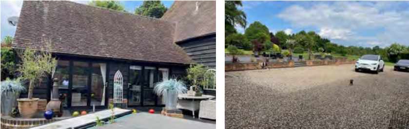
Existing Materiality - West side of ailed barn with poorly aged windows, single storey extension, landscaping with existing hard-landscaping within private garden.
