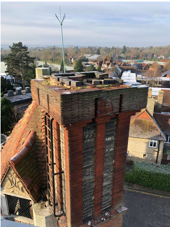
Tiling and brickwork loose to the top of the chimney.
