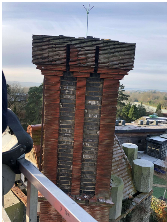
Significant loss of pointing
