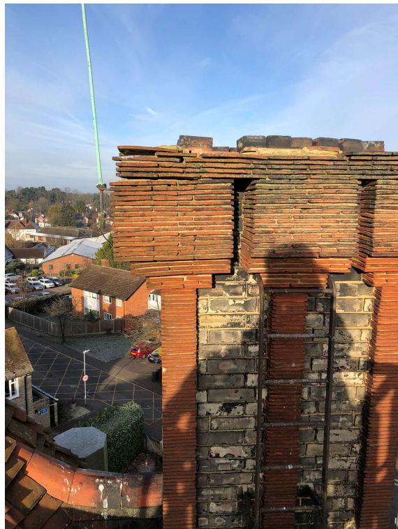
Loose corbel head and jacking caused by lightning conductor.
