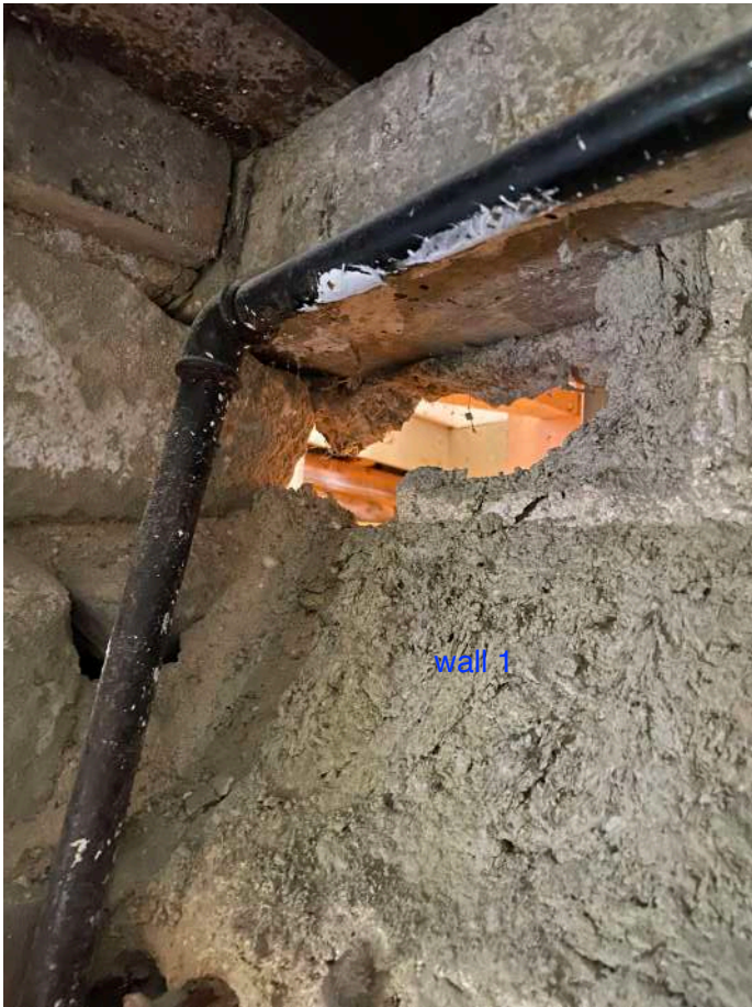
Void at top of Wall 1
