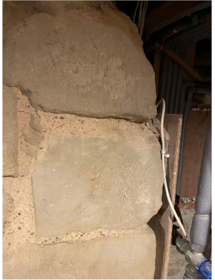
Wall 2 loose mortar
