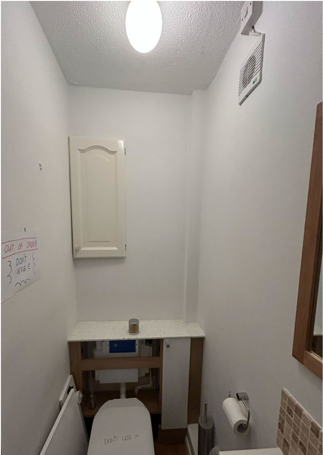
Ground Floor Toilet out of order
