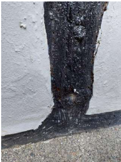
Figure 9. Bottom of stud appeared decayed and infilled with painted render
