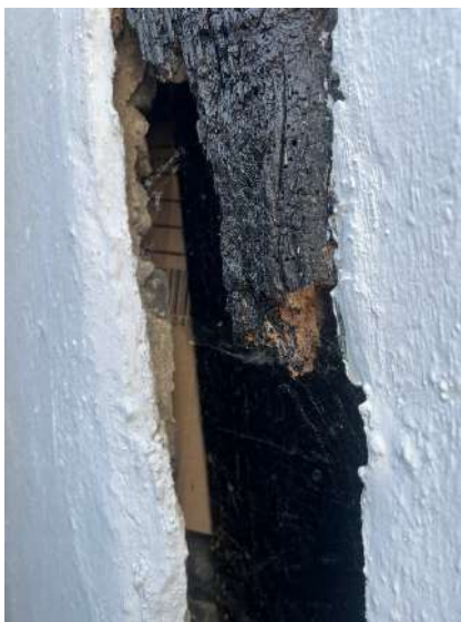
Figure 8. Stud is missing from wall plate up to 1m above wall plate
