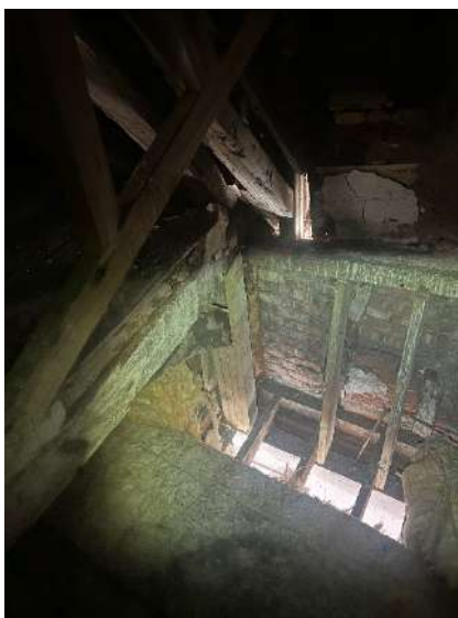
Figure 7. Rotten end of truss supported off timber post
