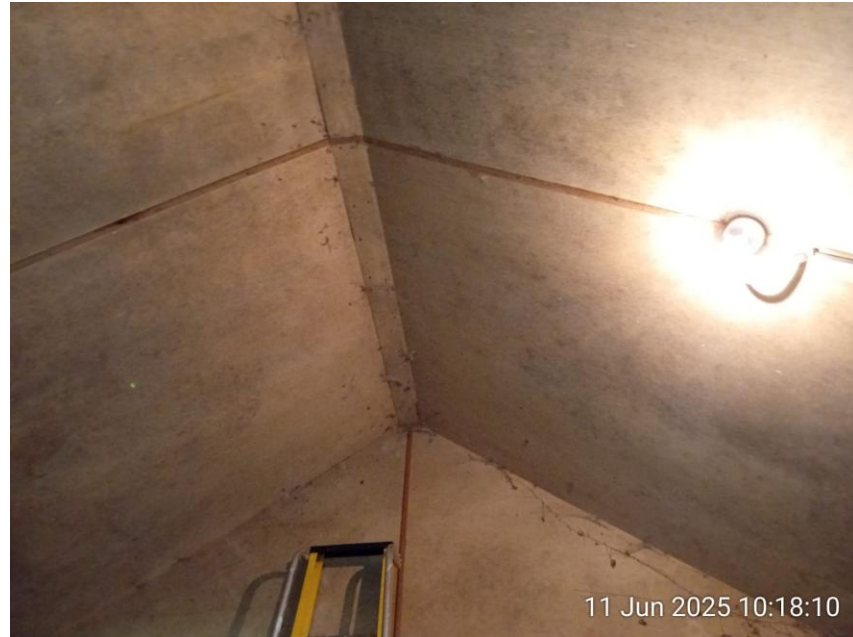
Figure 4: Example of boarded interior of B1
