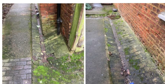
Damp in the base of the south wall caused by the drainage channel
