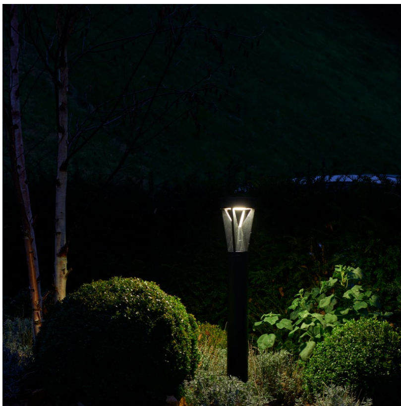
Plate 2: DW Windsor Pharola DS1 LED Bollard installed around a car park
