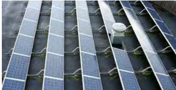
Rooftop Solar Panels
