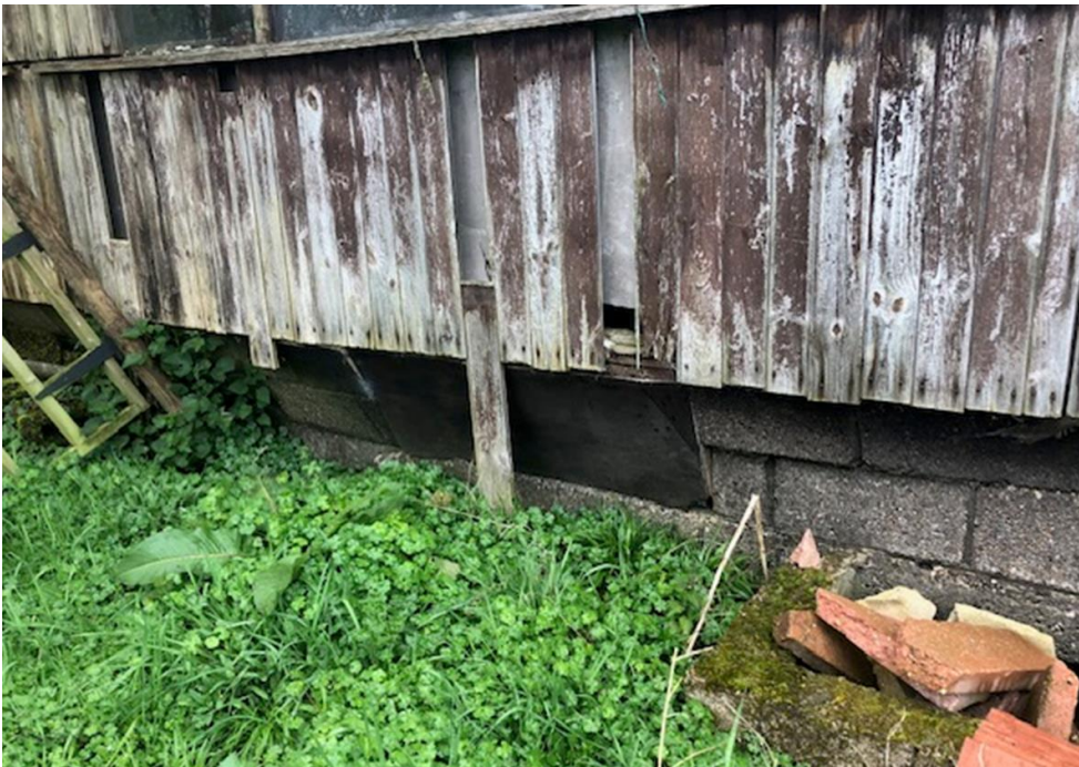
Damage to southern wall.
