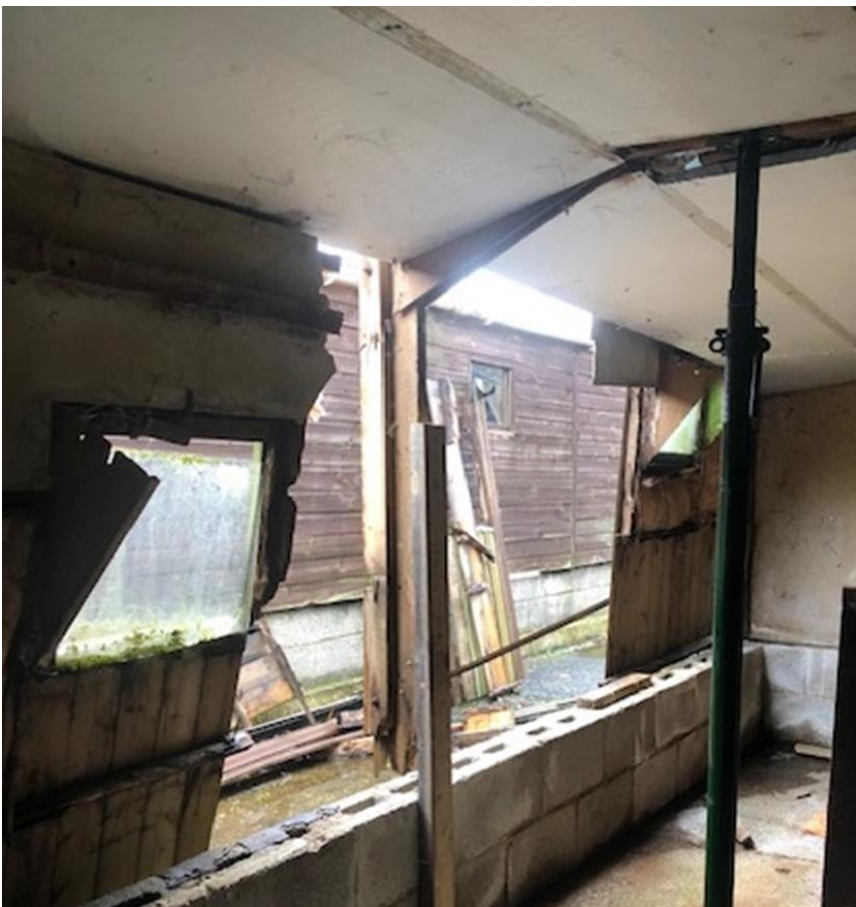
Collapsed wall to rear northern elevation.
