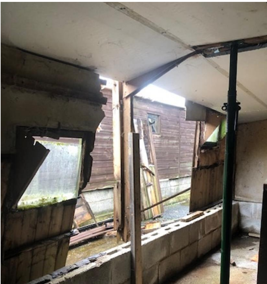
Collapsed wall to rear northern elevation.
