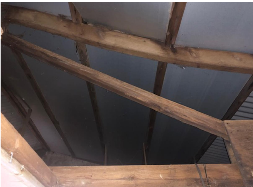
Failed rafter member in truss near front of building.
