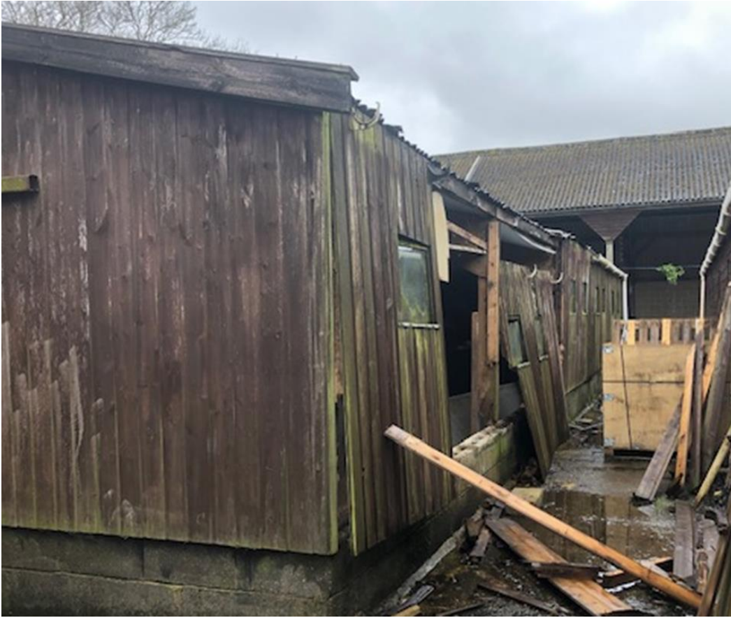
Collapsed wall to rear northern elevation viewed externally.
