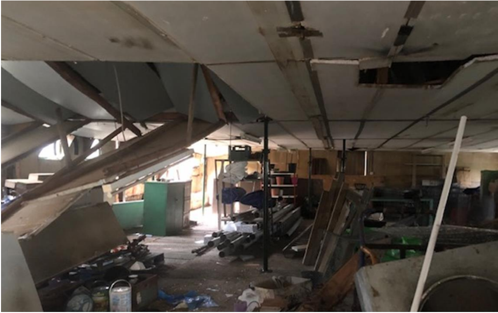
Failed roof near rear of building.
