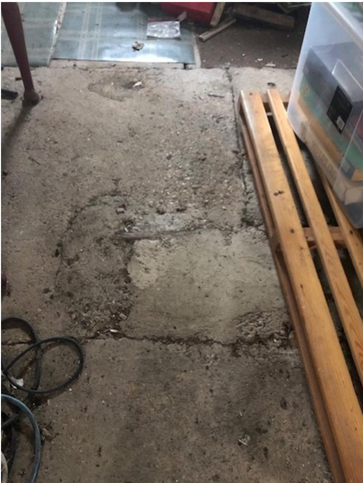
Uneven flooring and opened joints around suspected repairs.
