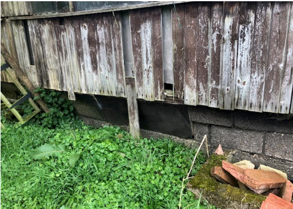
Damage to southern wall.
