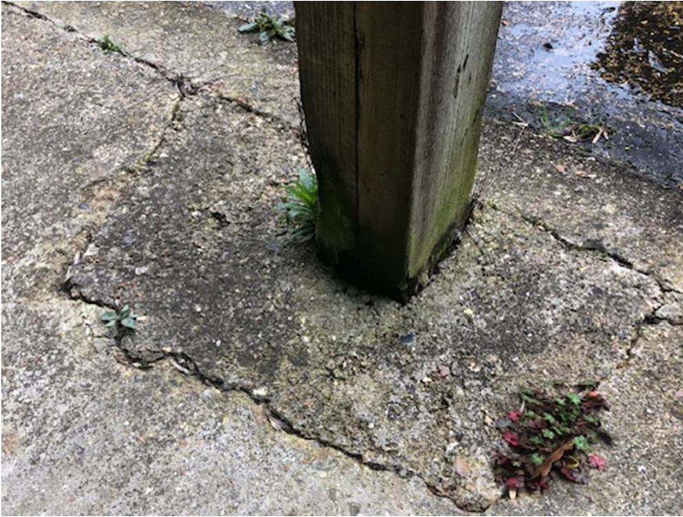
Timber post at ground level.
