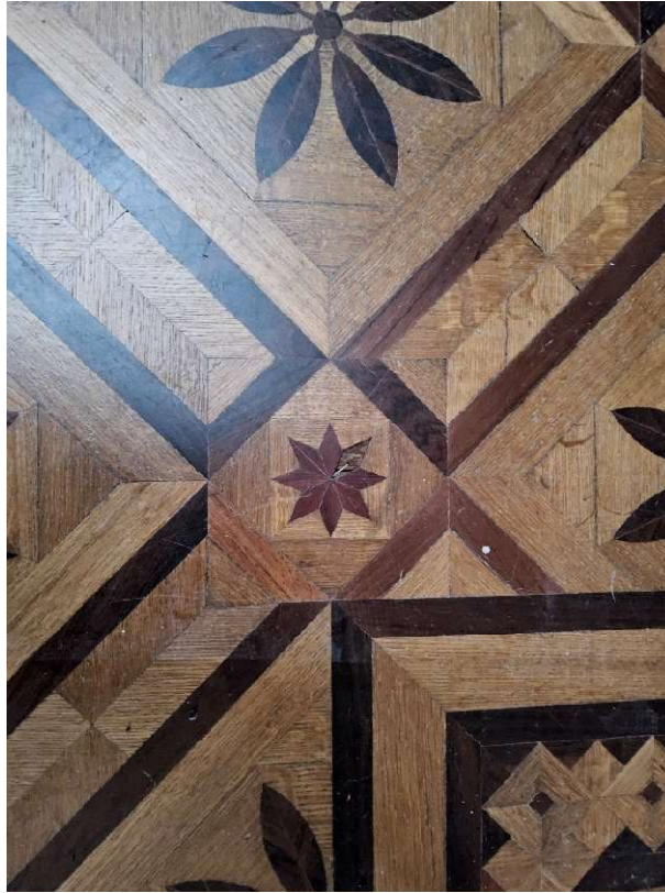
Sections of veneer missing
