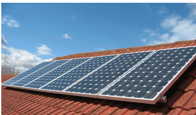
Figure 2: Monocrystalline PV arrays
