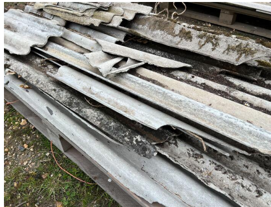
Potential asbestos sheeting.
