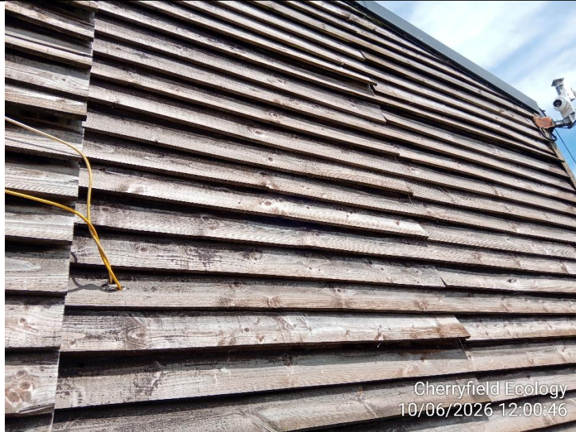
Figure 13: Lifted timber cladding.
