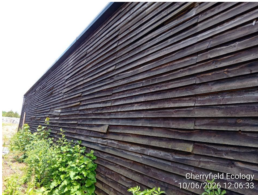
Figure 14: Lifted timber cladding.
