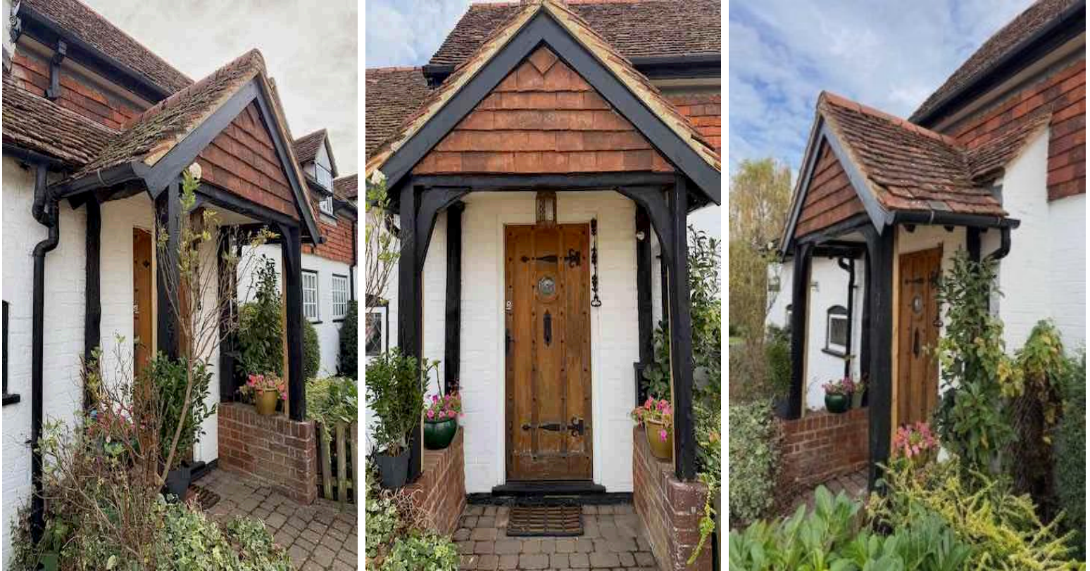
Quarter side and Front elevations of Porch, noting deflection at eaves level
