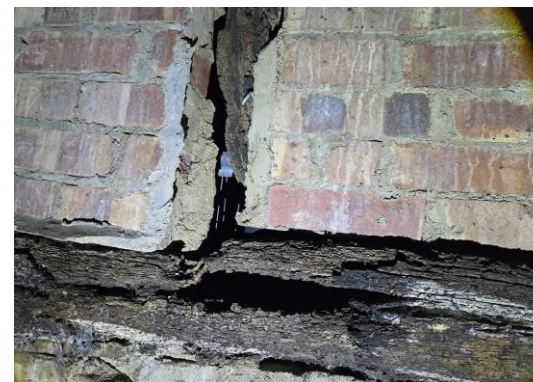
Gaps present throughout buildings
