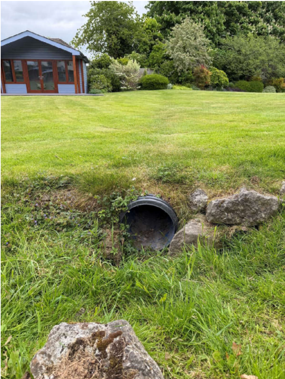
Photograph 4 – pipe in application site
