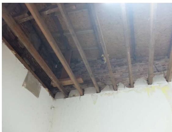
Fig.42 Roof structure exposed due to a leak in the SW corner
