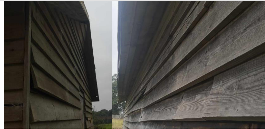
Figure 3. Two examples of warped exterior cladding, north and west elevations, respectively.
