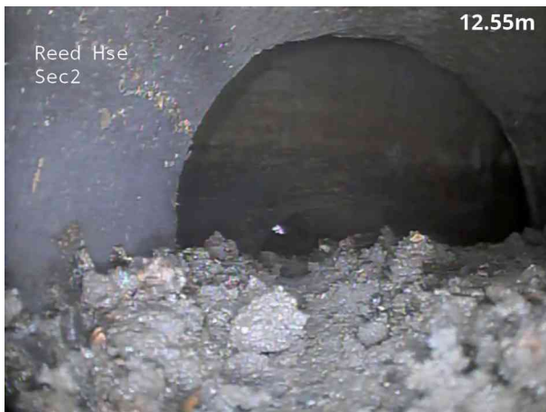
5, 00:01:19, 12.60 m Settled deposits, fine, 20% cross-sectional area loss, finish
