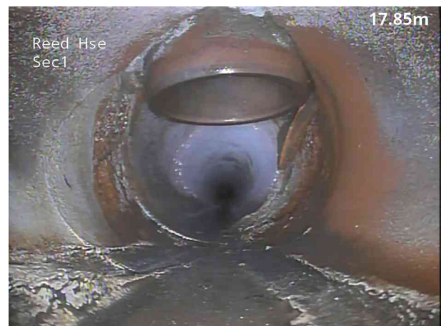
18, 00:12:12, 18.00 m Connection defective, connecting pipe is intruding at 12 o'clock, 150mm dia, intrusion: 25%
