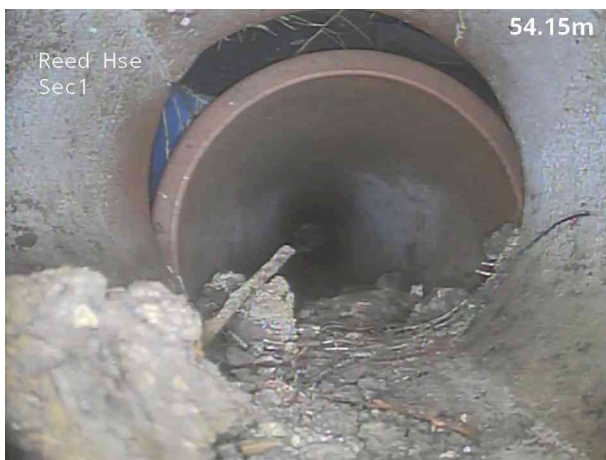
45, 00:07:49, 54.40 m Joint displaced, large
