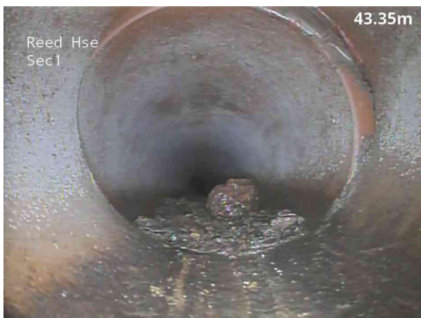
35, 00:09:18, 43.50 m Settled deposits, coarse, 20% cross-sectional area loss, start
