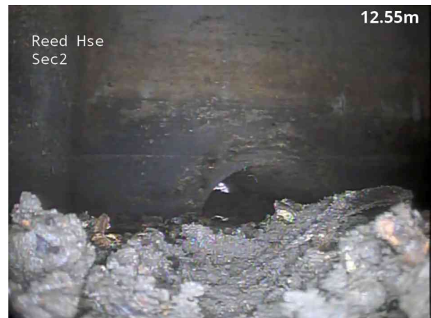
6, 00:01:19, 12.60 m Settled deposits, fine, 20% cross-sectional area loss, finish
