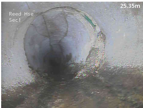
23, 00:11:21, 25.50 m Fracture, longitudinal at 12 o'clock, start
