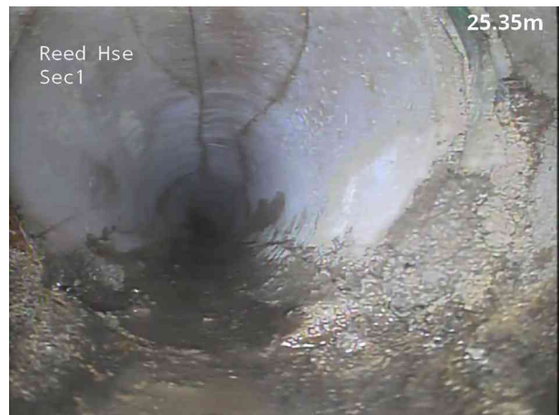
24, 00:11:21, 25.50 m Fracture, longitudinal at joint at 11 o'clock
