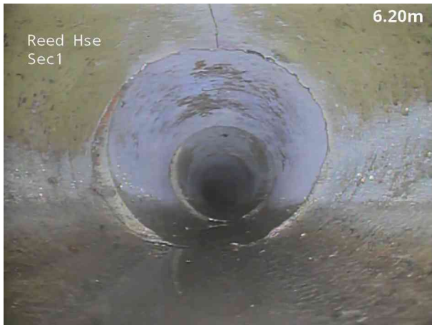
9, 00:13:35, 6.40 m Fracture, longitudinal at 12 o'clock, finish
