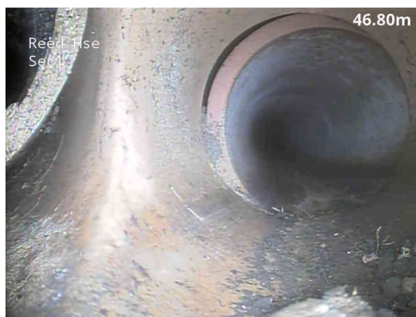
40, 00:08:41, 47.00 m Joint displaced, medium
