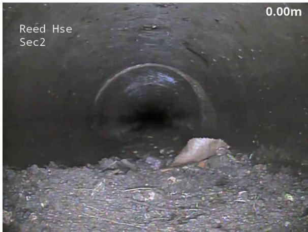
3, 00:00:09, 0.00 m Settled deposits, fine, 25% cross-sectional area loss, start
