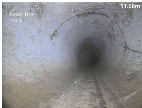
42, 00:08:08, 51.80 m Fracture, longitudinal at 9 o'clock, finish
