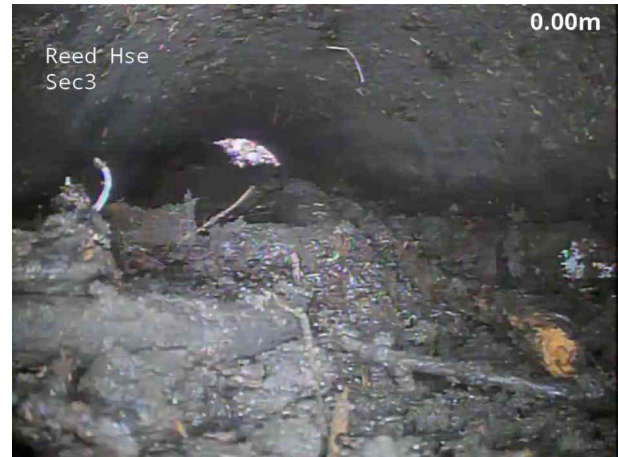
2, 00:00:35, 0.00 m Settled deposits, coarse, 75% cross-sectional area loss, start
