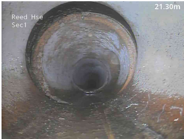
19, 00:11:54, 21.50 m Open joint, large
