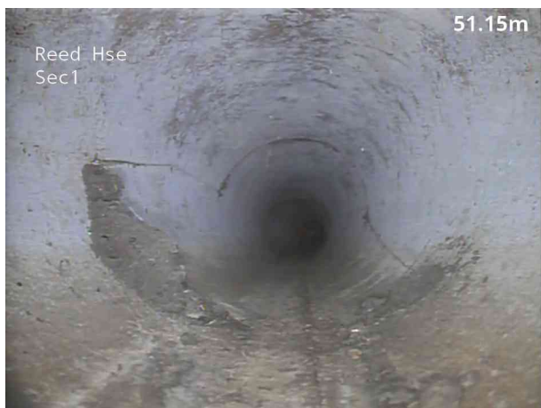
41, 00:08:03, 51.30 m Fracture, longitudinal at 3 o'clock, start
