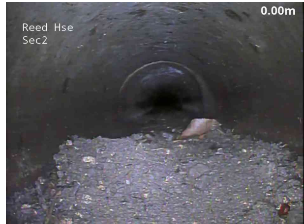
2, 00:00:09, 0.00 m Settled deposits, fine, 25% cross-sectional area loss, start
