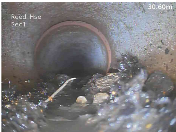
31, 00:10:22, 30.60 m Settled deposits, coarse, 25% cross-sectional area loss, change
