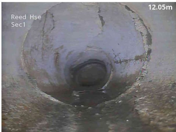
11, 00:13:10, 12.20 m Fractures, multiple at joint from 12 o'clock to 12 o'clock
