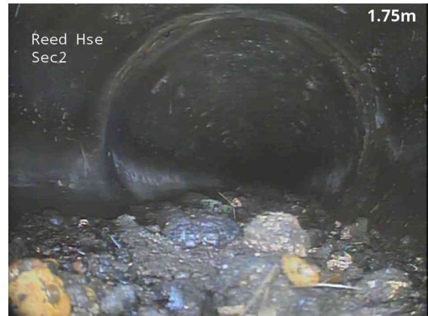
4, 00:00:29, 1.80 m Settled deposits, fine, 20% cross-sectional area loss, change
