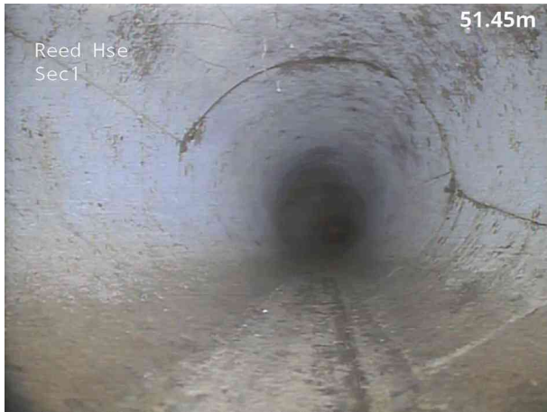
43, 00:08:08, 51.80 m Fracture, circumferential from 10 o'clock to 4 o'clock
