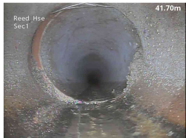
34, 00:09:34, 41.80 m Joint displaced, medium
