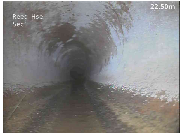
22, 00:11:37, 22.60 m Fracture, longitudinal at 9 o'clock, finish
