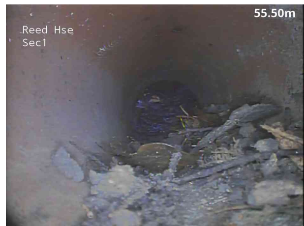
46, 00:07:34, 55.50 m Settled deposits, coarse, 20% cross-sectional area loss
