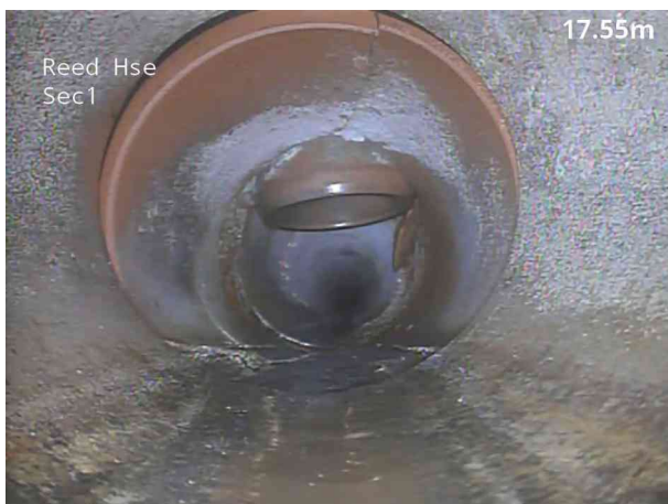
17, 00:12:17, 17.80 m Fracture, longitudinal at joint at 1 o'clock
