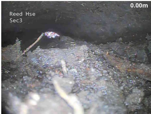
1, 00:00:35, 0.00 m Settled deposits, coarse, 75% cross-sectional area loss, start
