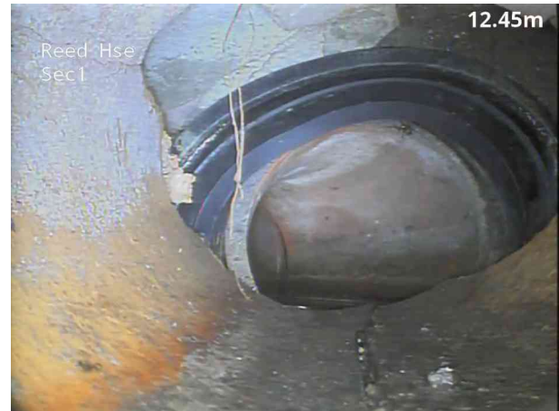
14, 00:12:48, 12.50 m Joint displaced, large
