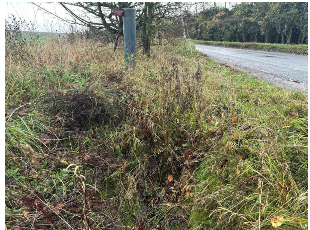
Headwall 6? No pipe visible
