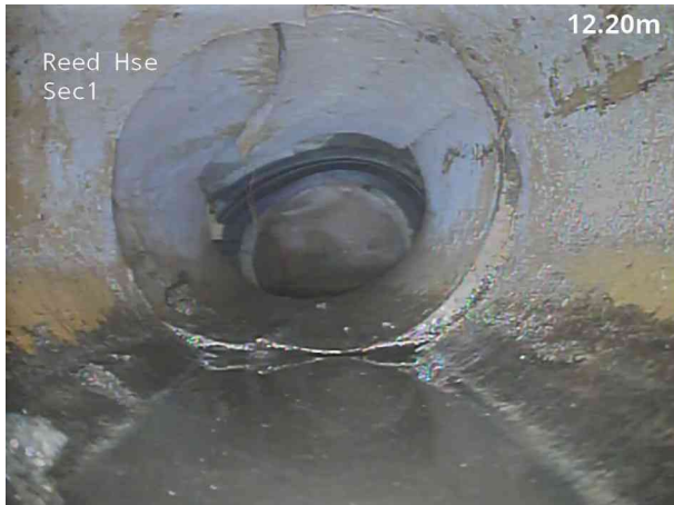
13, 00:13:01, 12.40 m Deformed sewer or drain, 10%
