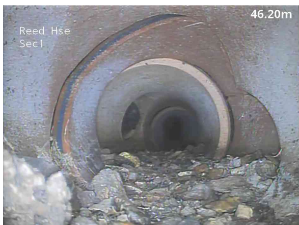
37, 00:08:56, 46.40 m Broken pipe from 12 o'clock to 12 o'clock
