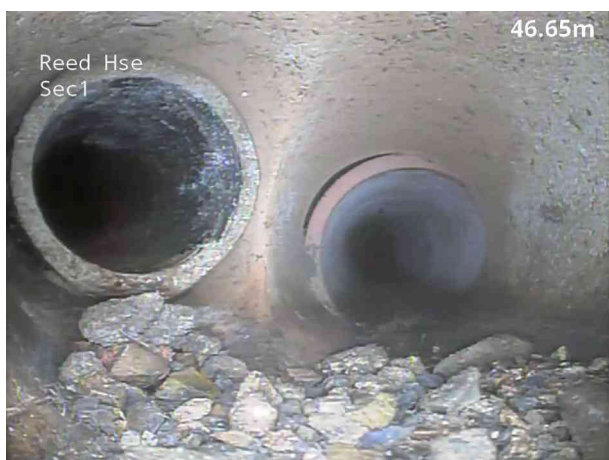
39, 00:08:49, 46.80 m Settled deposits, coarse, 20% cross-sectional area loss, finish
