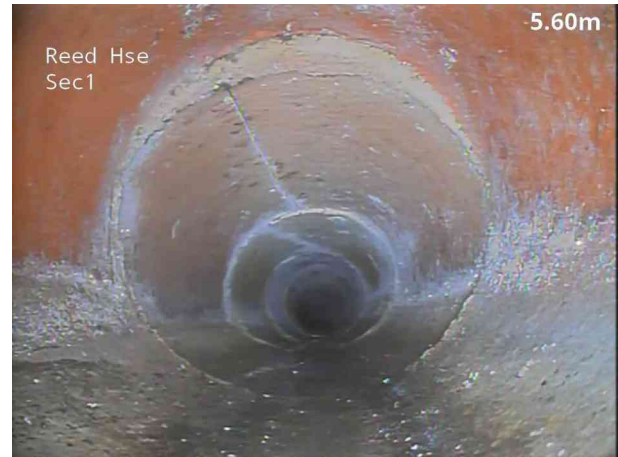
8, 00:13:35, 5.60 m Fracture, longitudinal at 12 o'clock, start
