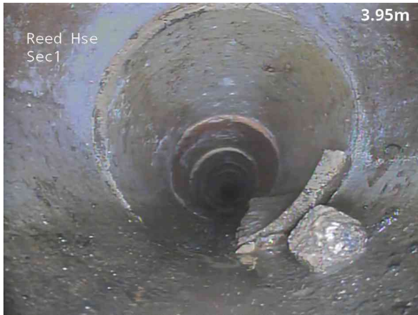
7, 00:13:51, 4.00 m Settled deposits, coarse, 10% cross-sectional area loss
