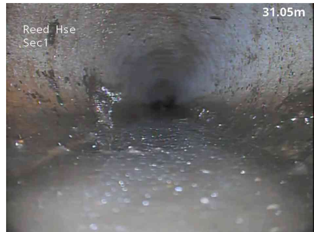
32, 00:10:17, 31.00 m Settled deposits, coarse, 25% cross-sectional area loss, finish
