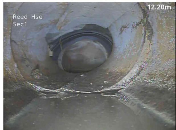
12, 00:13:01, 12.40 m Deformed sewer or drain, 10%
