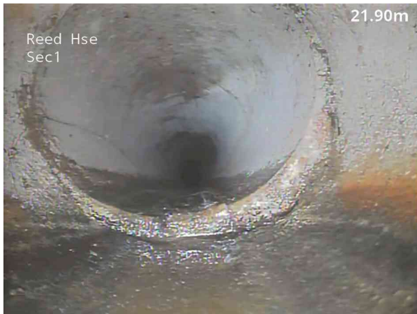
21, 00:11:43, 22.00 m Fracture, longitudinal at 9 o'clock, start
