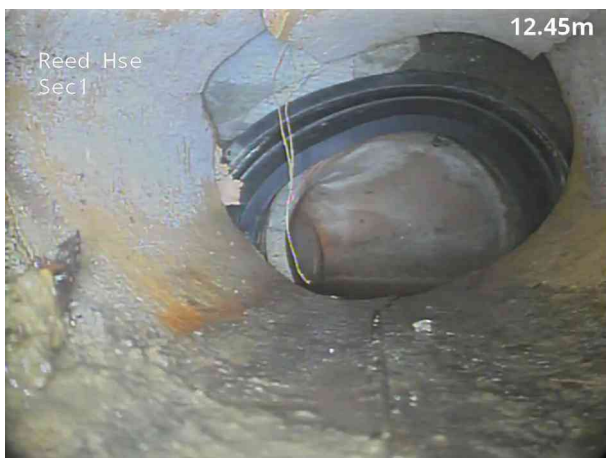
15, 00:12:54, 12.50 m Broken pipe at joint from 9 o'clock to 3 o'clock
