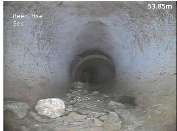
44, 00:07:52, 54.00 m Settled deposits, coarse, 10% cross-sectional area loss
