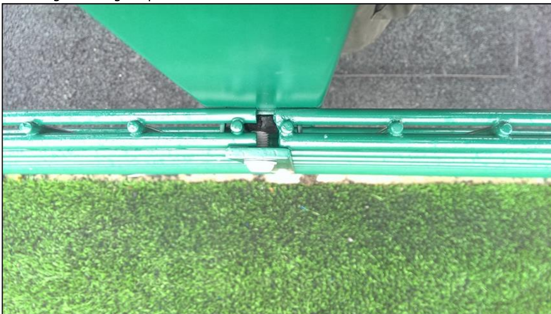
Figure 9: Image showing neoprene isolators
