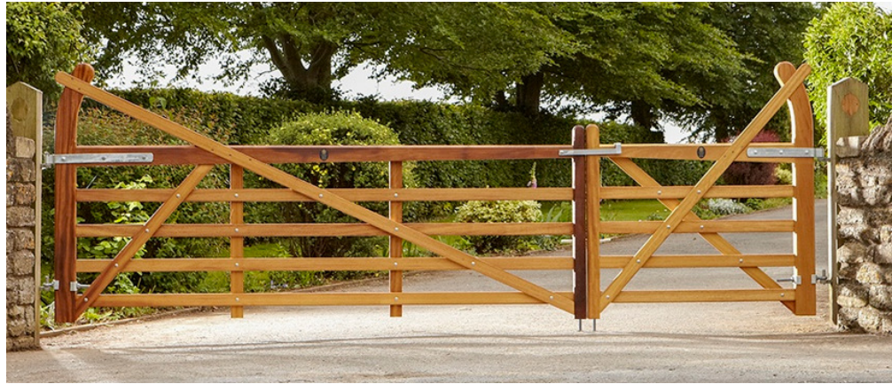
pedestrian and vehicular timber gate Condition 3
