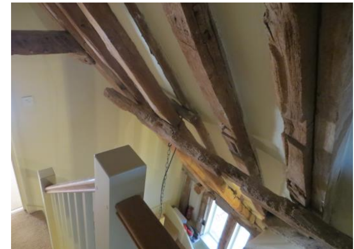
Figure 4.181: Showing an incomplete purlin and the partnered rafter used in this part of the building.
