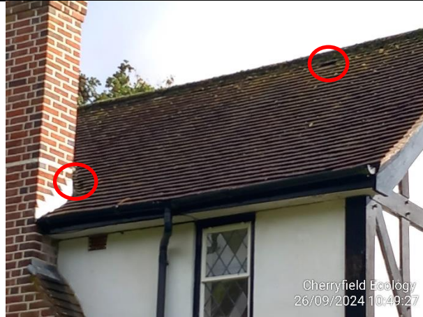
Figure 9: Example of gaps in the roofing tiles
