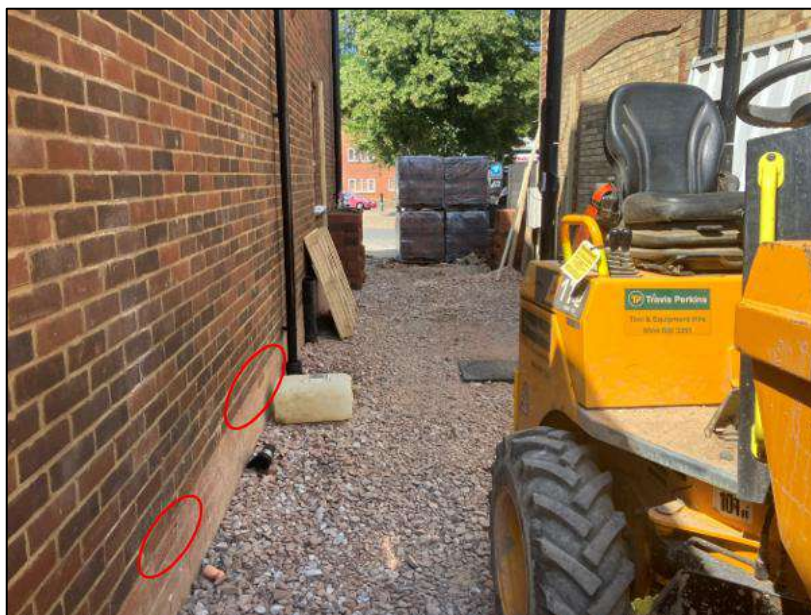
Figure 8-B: Example of external vents (highlighted in red)
