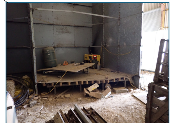
STANDBY GENERATOR INSIDE GRAINSTORE
