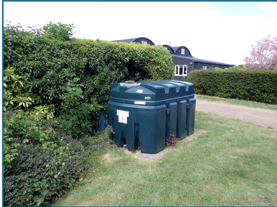
HEATING OIL TANK OFF SITE
