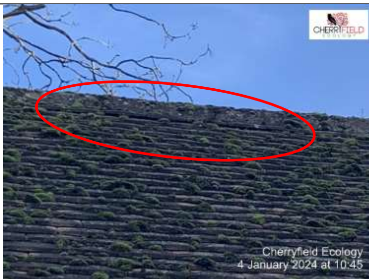
Figure 30: Lifted clay tiles above garage attached to B1.
