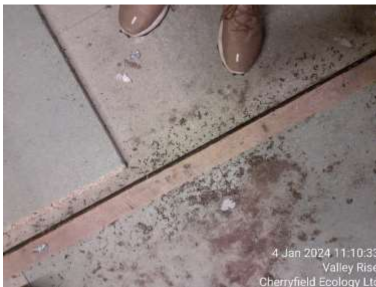
Figure 29: Bat droppings found within the loft in the main section on B1.
