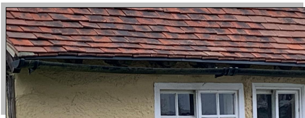
Poorly fitted gutter on north elevation
