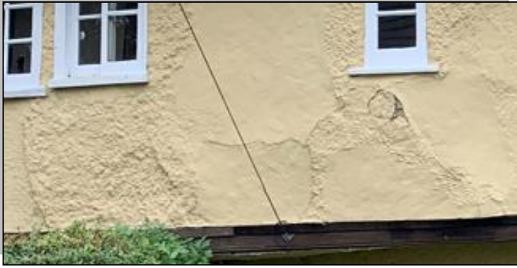
Example of current loose and unstable cementitious render to North, East and West elevations
