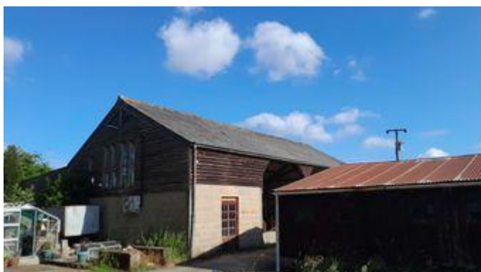
Suspected asbestos roof on barn in east of site.
