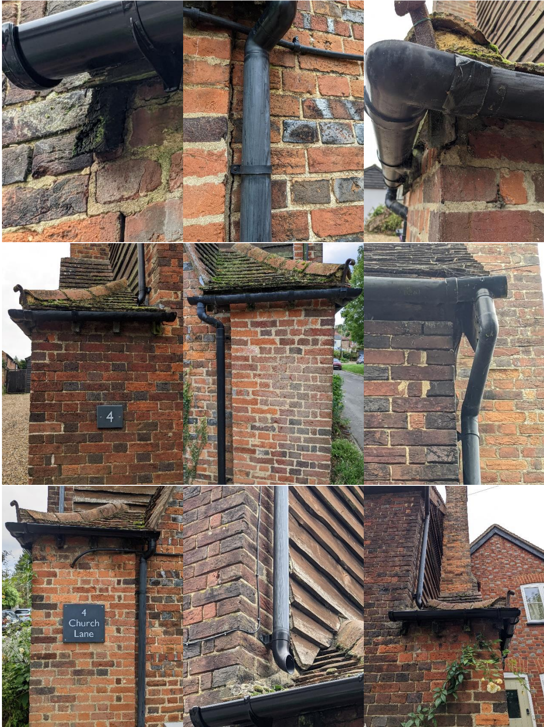
Fig 2 – Showing Defects in Current System
