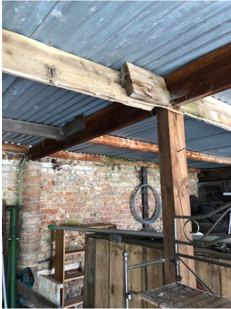
Photo – 8: Twisted & Warped Timber Roof Purlins
