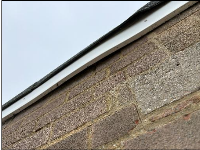
Photograph 12 Small gaps under fascia on north-western elevation of B1b – fully inspected with endoscope
