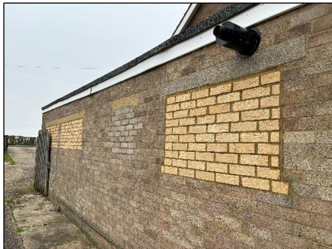
Photograph 11 Small gaps under fascia on north-western elevation of B1b – fully inspected with endoscope
