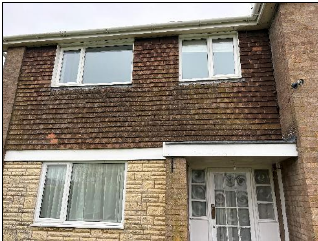
Photograph 13 Gap between hanging tiles and brickwork on right hand side – where bat was seen to emerge
