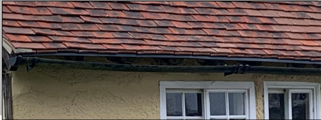
Poorly fitted gutter on north elevation
