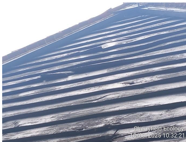
Figure 21: Example of the lifted timber shiplap on B2
