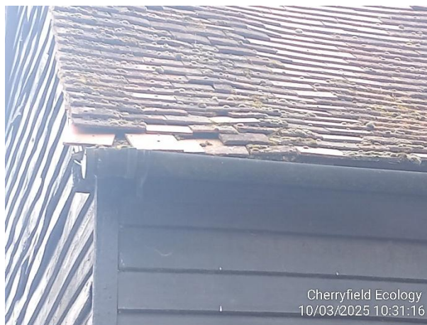
Figure 20: Example of lifted clay tiles on B2
