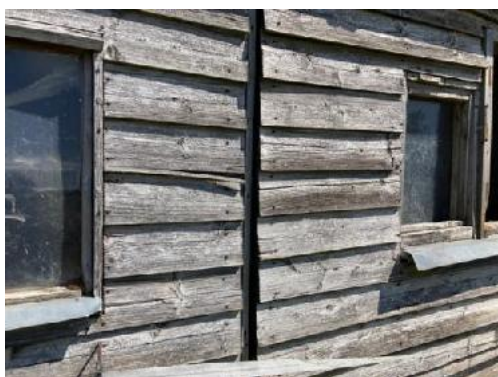
Photograph 11: Example of lifted wood cladding
