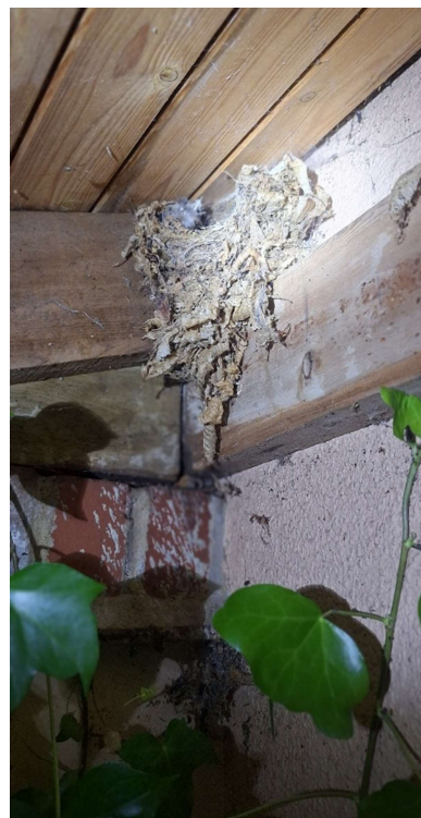
Photograph 7. Bird nest, Building B
