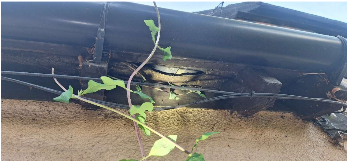
Photograph 10: Holes in soffits, eastern aspect of Building A
