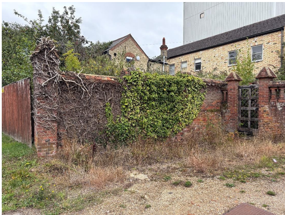
Boundary wall viewed from roadside. Significant ivy growth on the wall
