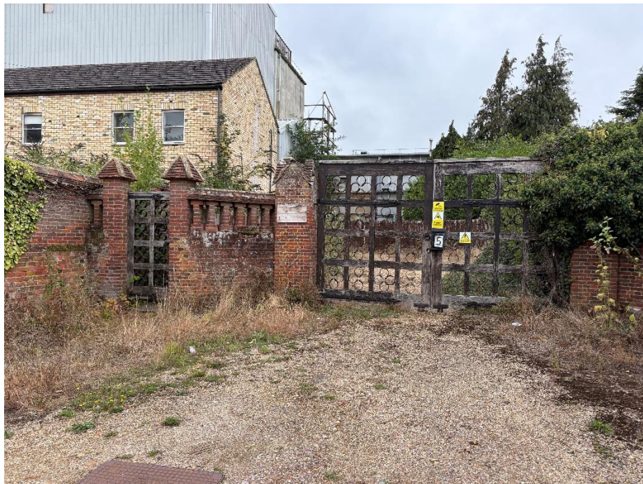
Entrance gate, Piers and wall. Ivy growth on Northern gate pier
