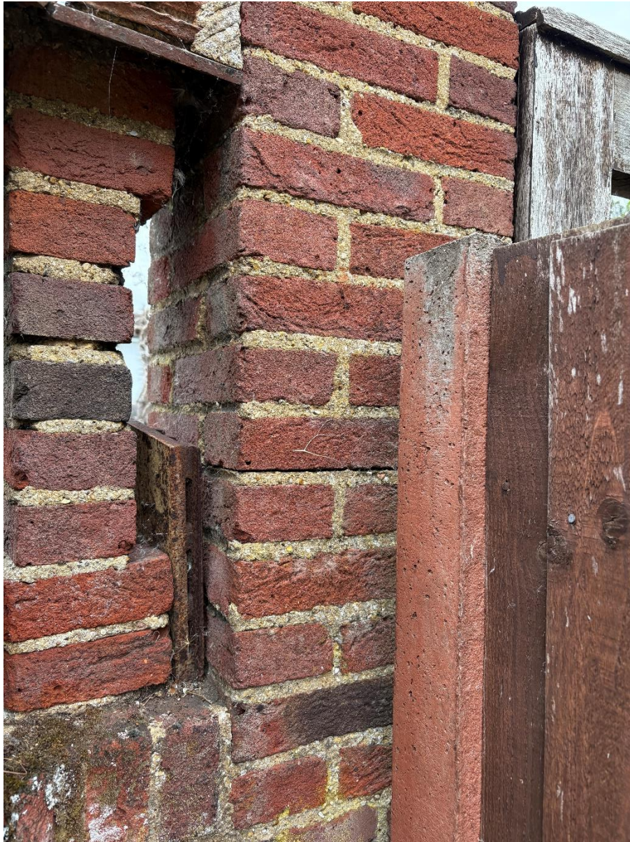
Horizontal crack in pier to pedestrian gate pier
