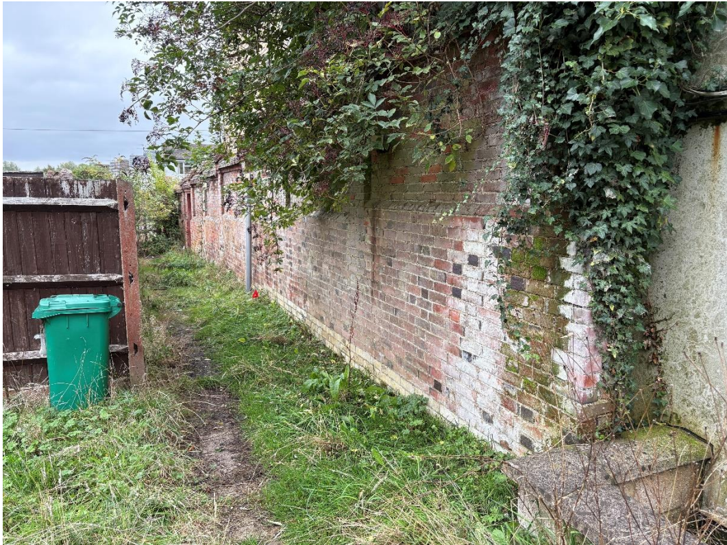
Ivy and moss growth with water staining to the wall from missing rainwater pipe to mill building
