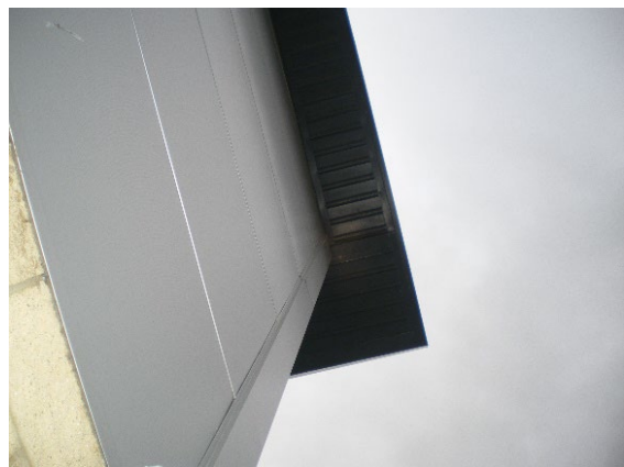
Feature 1: Gap behind the metal cladding, roof level. South elevation
