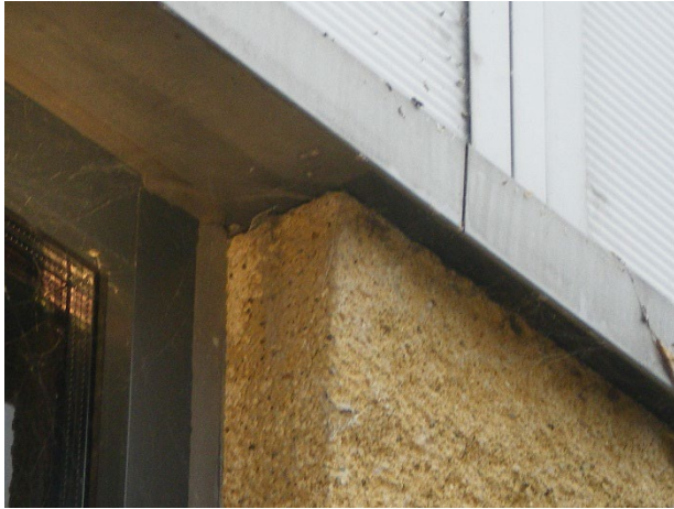
Feature 9: Gap between wall and metal cladding, left of the large window.
