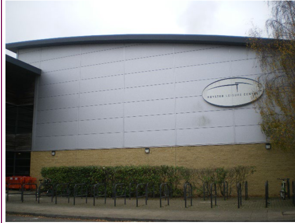
Feature 6: Gap between wall and roof edging along whole length. South, on west elevation
