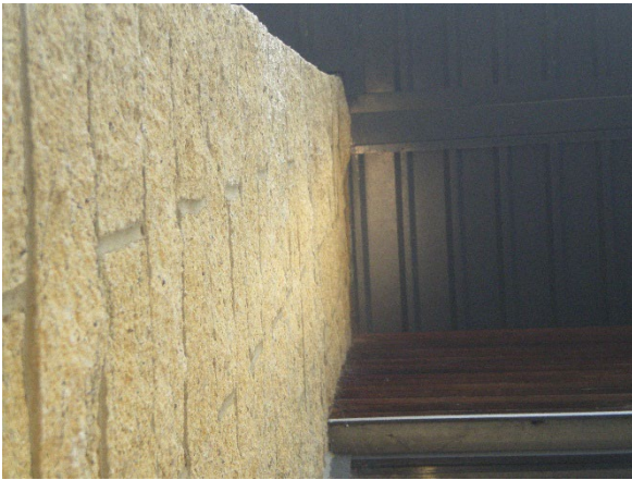
Feature 7: On the corner of the main entrance, gap between the top of the wall and roof. All along the brick work. North elevation
