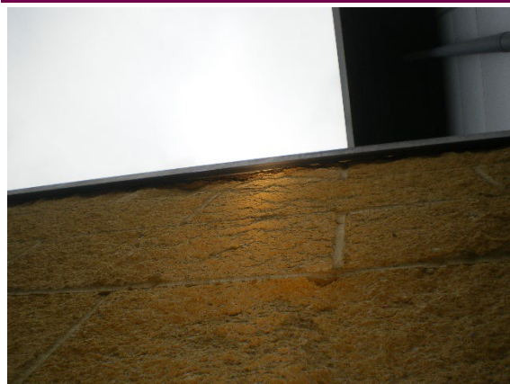
Feature 3: Gap behind the metal cladding, roof level. South, on west elevation
