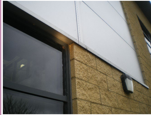
Feature 8: Gap between wall and metal cladding, right of the large window. North elevation
