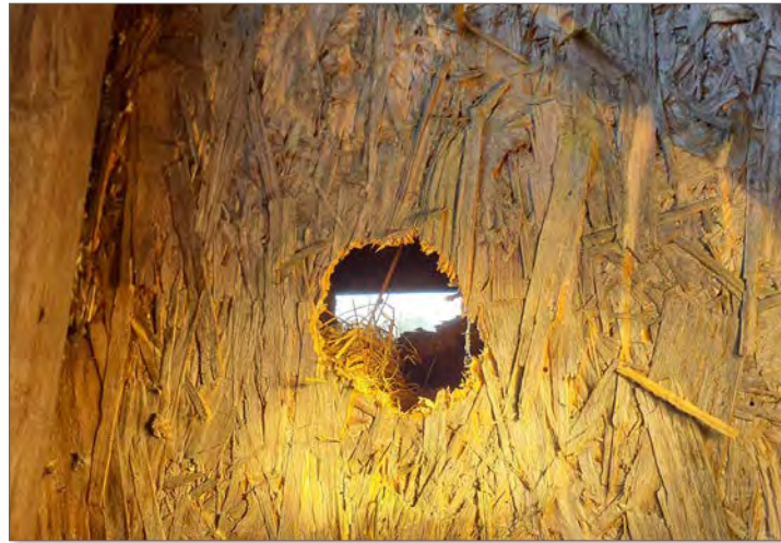
Building 1 Hole on southern interior wall with nest. Photograph taken 04/12/2024.
