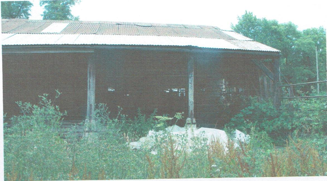
PHOTO No.14 Building B8 open timber frame with some metal support (assumed repairs), wiggly tin roof. Poor condition
