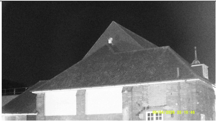
Surveyor IR image: Rear elevation - Finish
